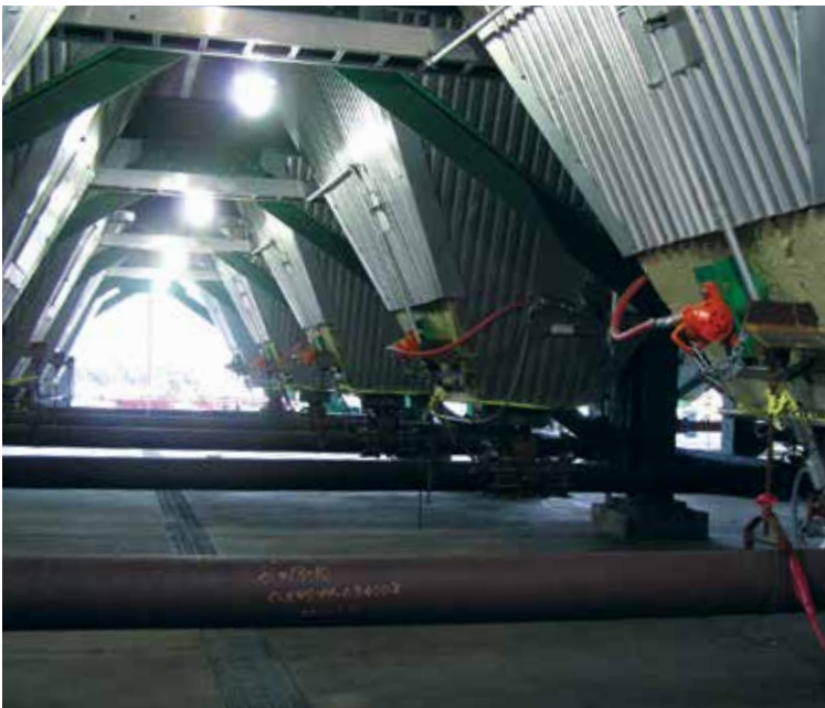
Above: The patented SVR design (page 30-31) shown in the dust collectors of this power plant, have a dB reading of 95-110. They are also available in a silent version which brings the dB down to 80-85.
