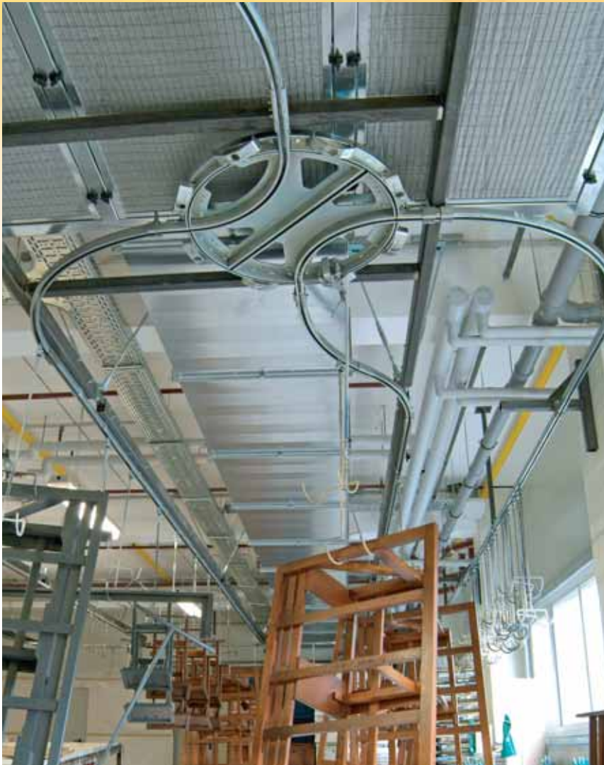
Overhead conveyor system with Müsing spider assembly.
