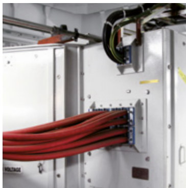
Generators and propulsion system: Roxtec seals are adaptable to fit cables and pipes of different sizes.
