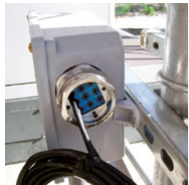
Telecom cabinet: The Roxtec RG M63 cable glands are weather, water, pest and dust tight.
