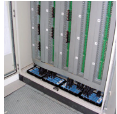
DCS/PLC and I/O marshalling cabinets: Roxtec solutions reduce required cabinet space, ensure functionality and provide capacity for additional cables.
