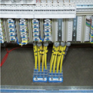
Transformers and switchgear: The Roxtec GHM solution provides protection to ensure operational reliability.
